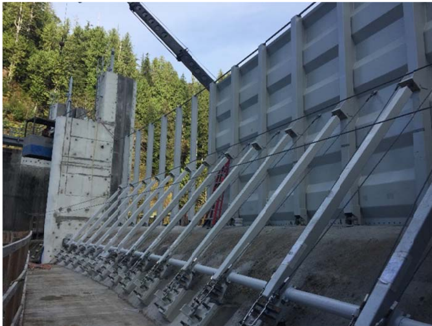
Flash Board Gate Installation
