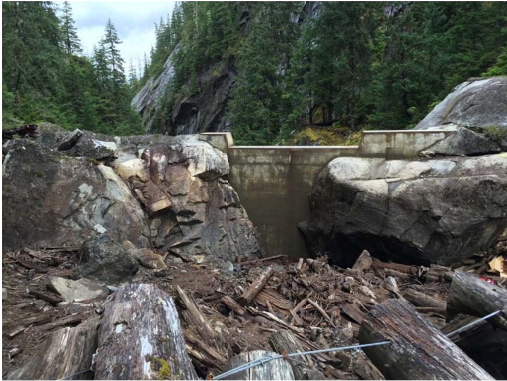
Tyee Lake Outlet Discharge Measurement Weir
