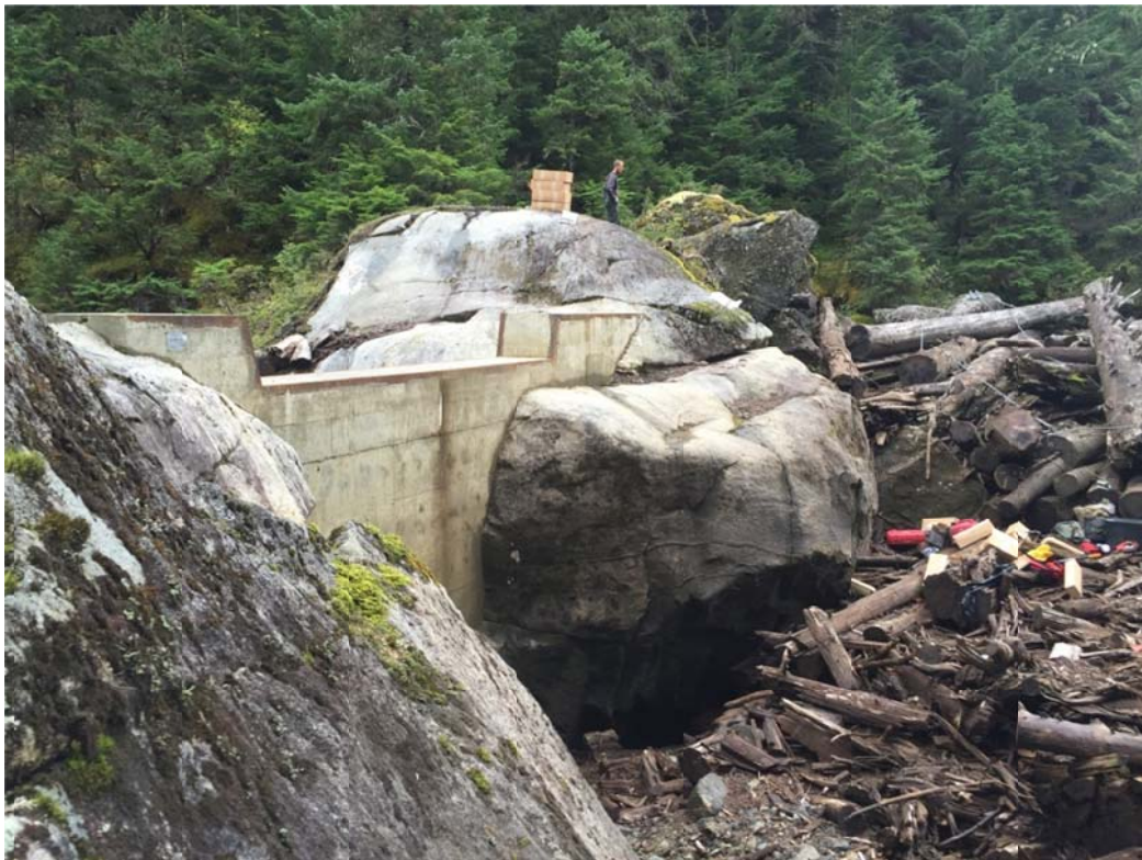
Right Abutment Upstream with Expandable Foam Boxes Staged for Placement on Downstream Side - Top of Weir Elevation 1396 Feet
