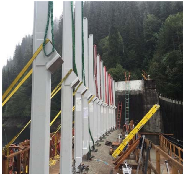
Flash Boards Columns Installed
