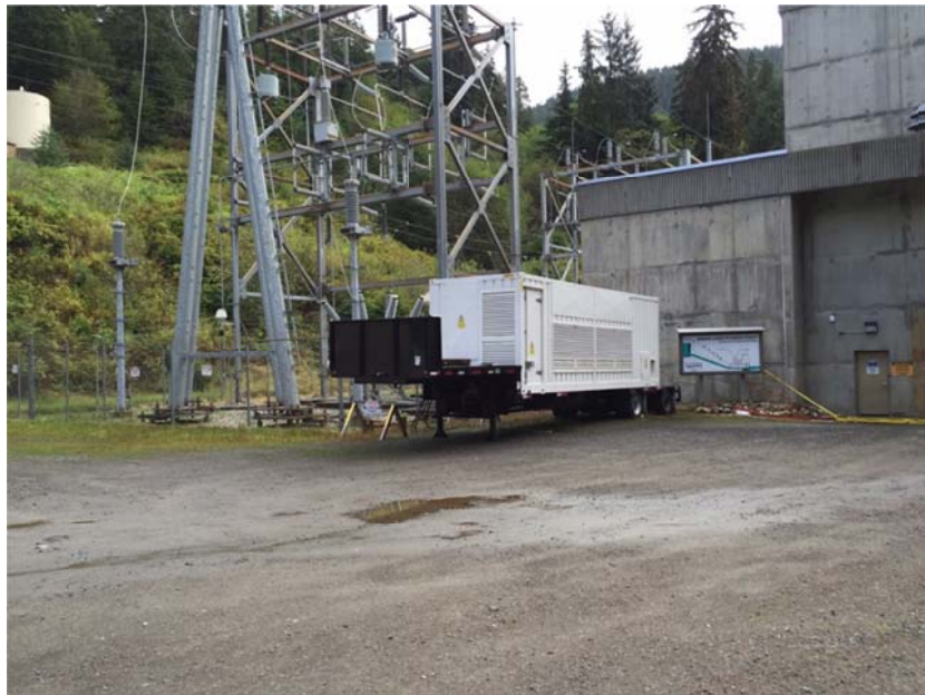
Crestchic 5 MW Load Bank at Swan Lake
