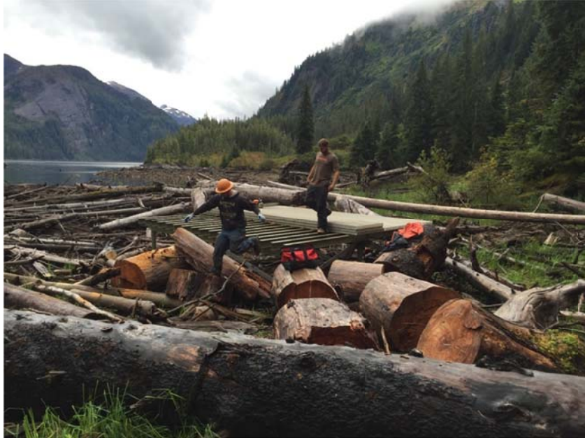
Disassembly of the Existing Helicopter Pad and Preparation for Transport by Helicopter
