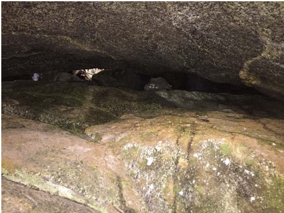
Typical Abutment Rock Voids Filled with Two-Part Expandable Foam During Phase 2 - Elevation 1395 Feet
