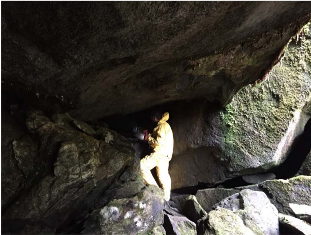
Voids and Fissures Along Downstream Sides of Right Abutment - Elevation 1378 Feet
