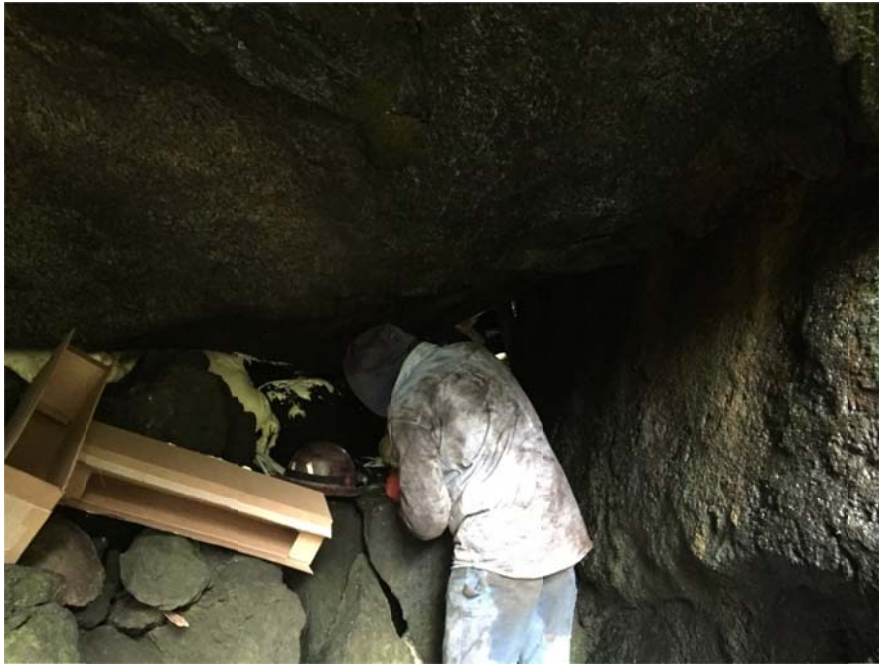
Expandable Foam Filling Voids of Right Abutment (Note Foam in Fissures) - Elevation 1380 Feet
