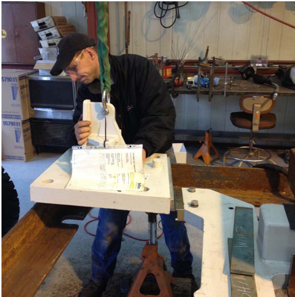
Swan crew member Rob Miller with fabricated jig for “kicker” column assembly
