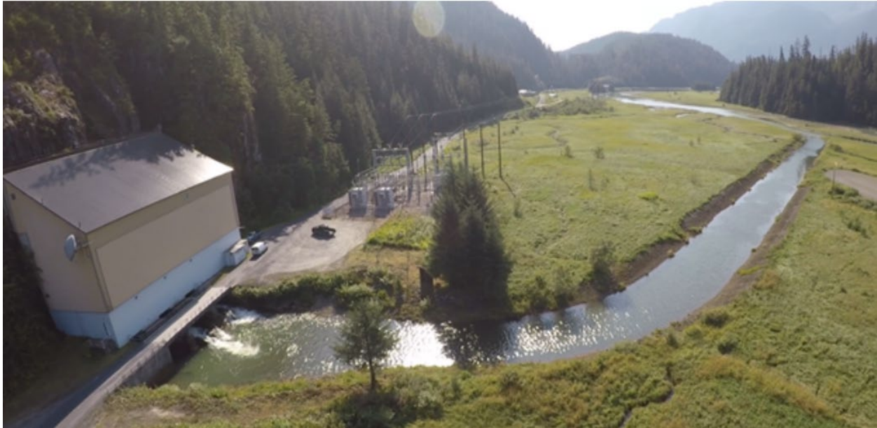
Photo 2-2 Typee Lake Powerhouse, Switchyard, and Tailrace.
