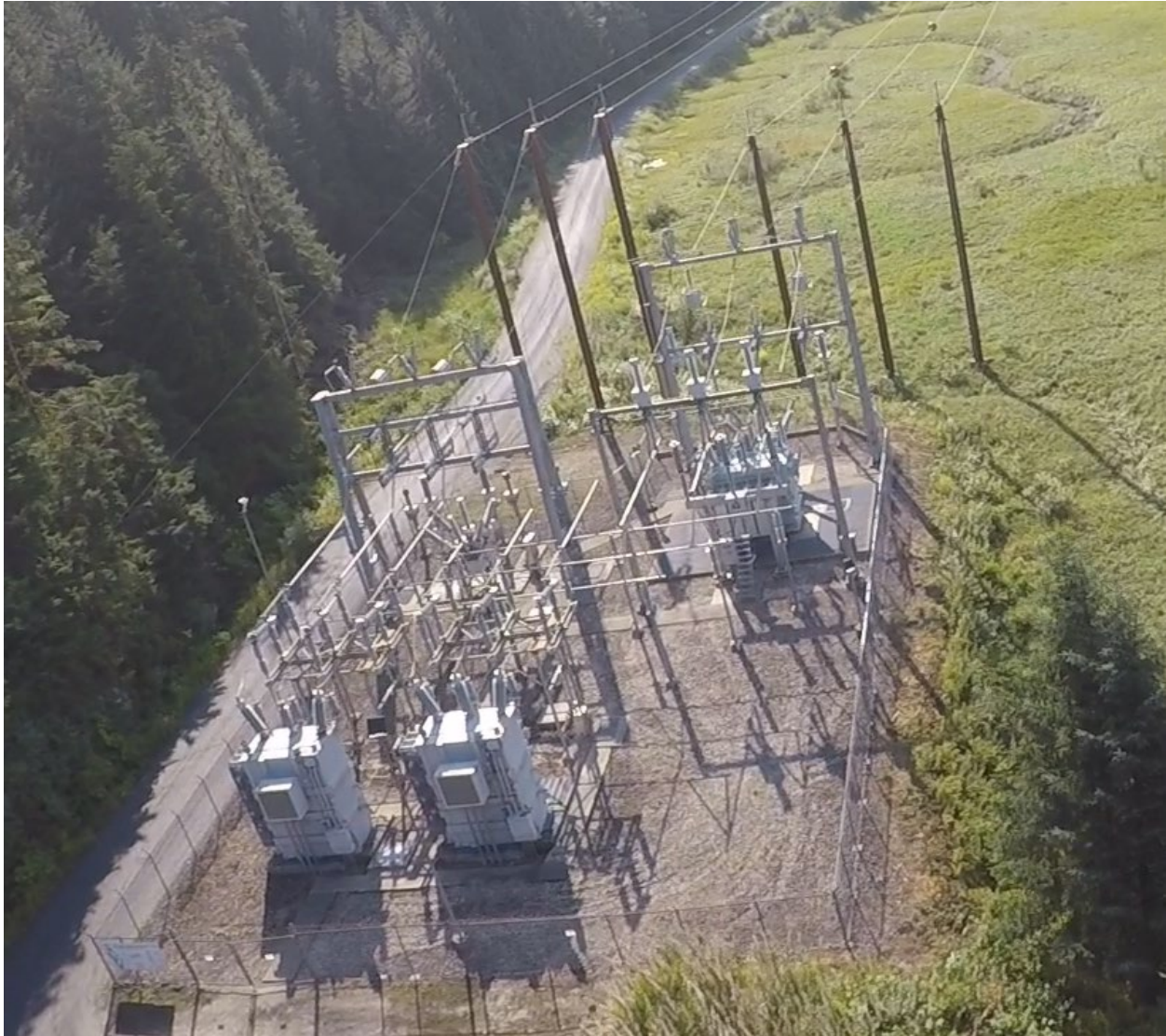
Photo 2-3 Tyee Lake Switchyard.
